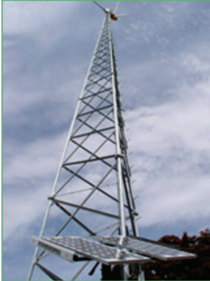
Sunderland Recycling Facility features a 10kW wind turbine that powers its offices.
