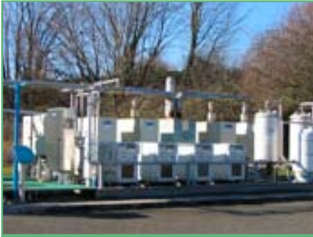
Microturbines at the Columbia Boulevard Wastewater Treatment Plant use biogas to generate electricity.
