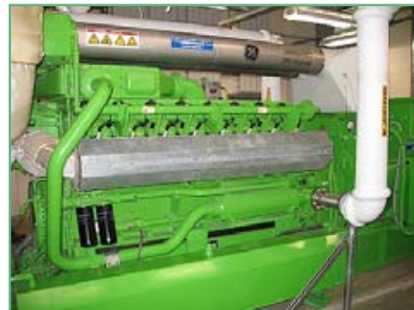
The City should recover the investment cost of the new reciprocating engine-generators within 12 to 15 years.
