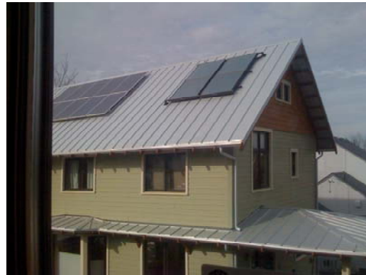
solar panels on a roof in NE Portland
